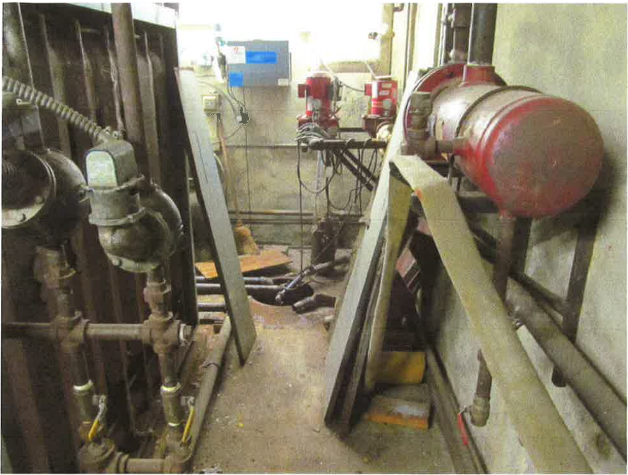
Boiler room sump pump - small pump for normal operations
